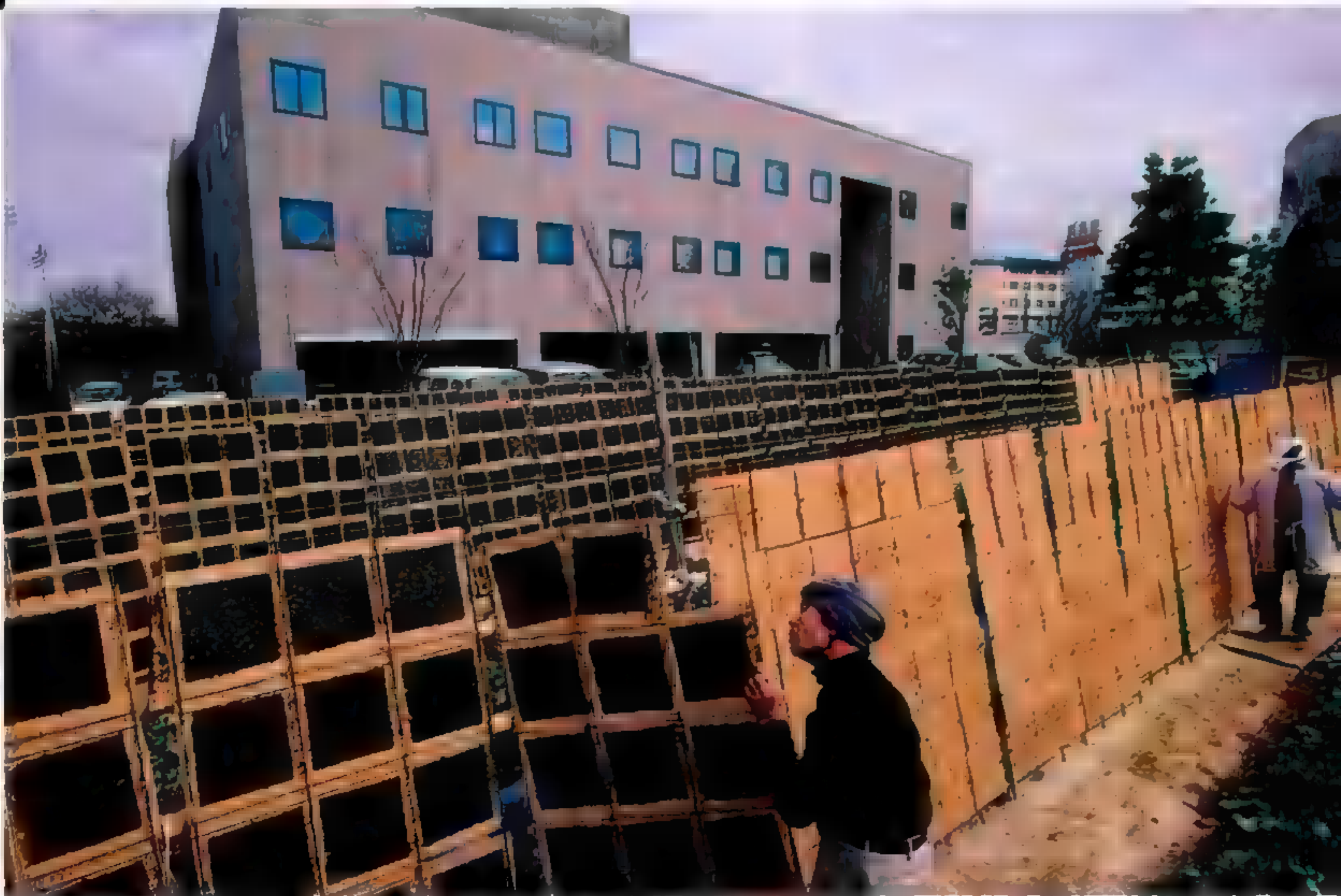
Workers teeter and toil on a giant gamble: the Yokohama convention center (top). While vacancy rates are high in some areas, falling land prices and government subsidies are fueling a construction boom. Traditional labor suits Kiichi Takiguchi (above), who collects and dries seaweed for sushi. But his work has gotten tougher: Landfill has moved the waterfront farther away.
